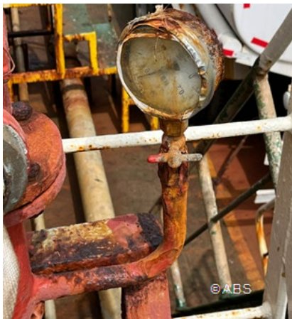
Faulty and damaged fire line pressure gauge with feed line and cock wasted
