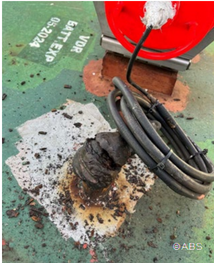
VDR (Voyage Data Recorder) cable penetration damage at monkey island
