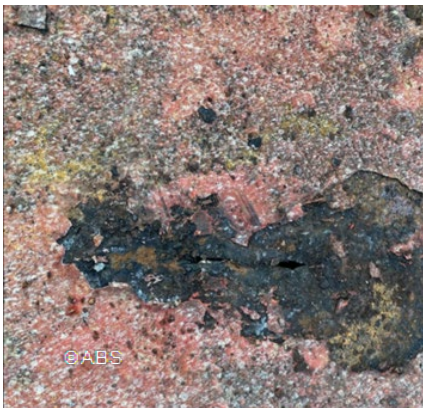
Main deck wasted with hole, next to hatch coaming in a bulk carrier
