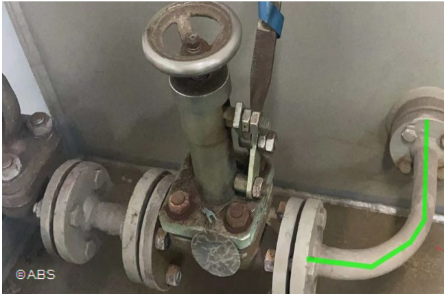
Emergency diesel generator quick closing valve-fitted with 250mm apart from tank, does not meet requirement
