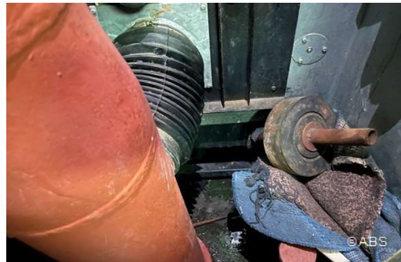
Sewage System flexible pipe leaking
