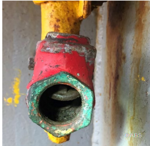
Cargo hold hatch coaming drainage pipe non- return valve stuck in open position
