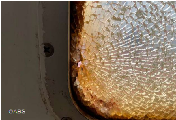
Accommodation window shattered with hole
