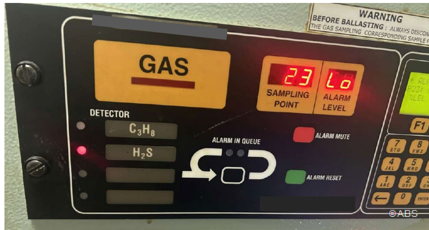
Fixed gas detection system failed to test hydrocarbon gas
