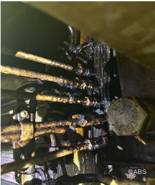
Excessive oil soaked around main engine service piping
