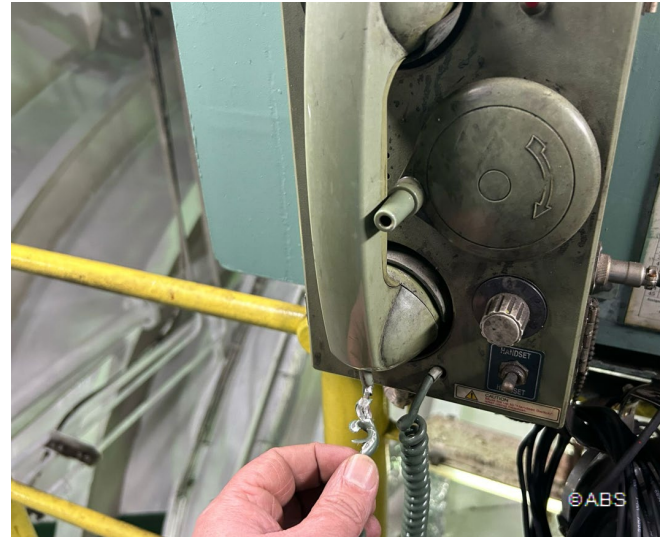
Emergency Generator Room telephone connection to hand set damaged
