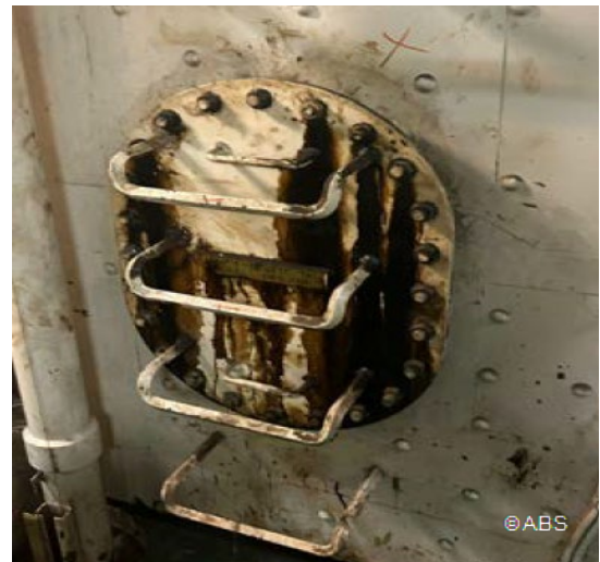
Fuel Oil Settling tank manhole cover leaking
