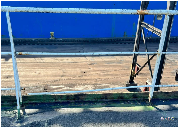
Broken guard rail
