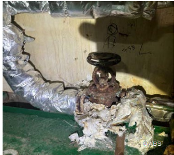
Steam heating valve for fuel oil tank, insulation deteriorated and not maintained
