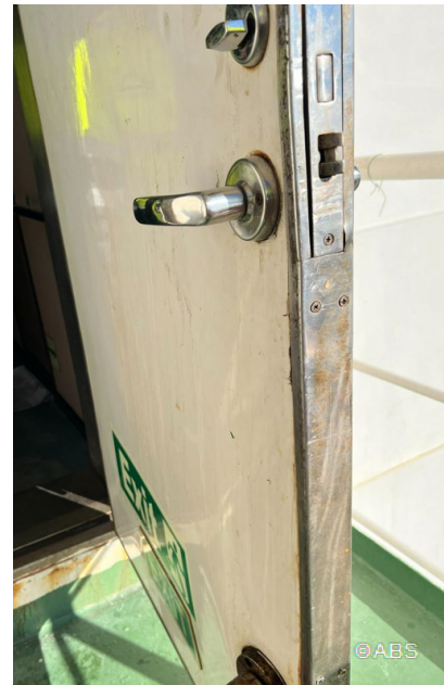
Accommodation door deformed
