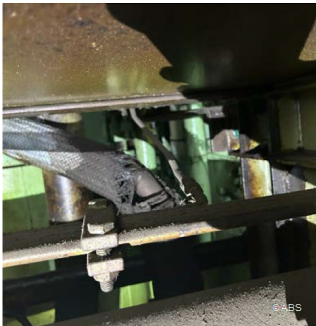
Main engine fuel pipe metallic sheathing damaged with missing part and not maintained
