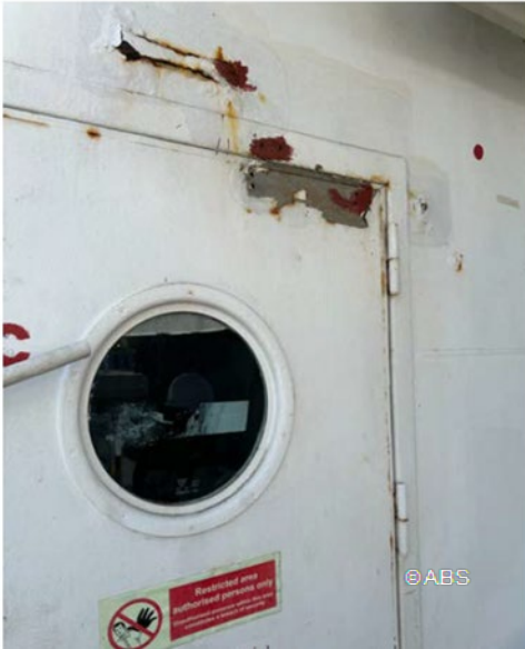
Missing self-closing hinge on accommodation door
