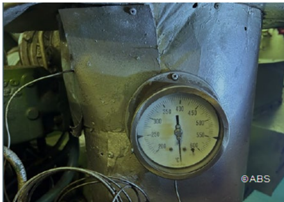
Defective diesel generator engine thermometer
