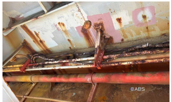
Loose and damaged cables on deck
