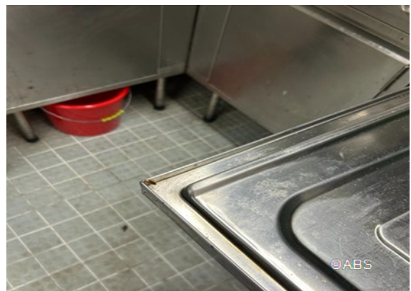
Bug infestation in galley store
