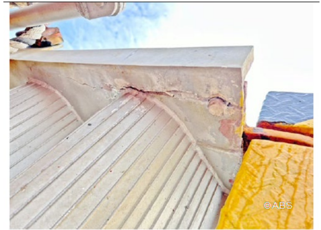
Damaged accommodation ladder
