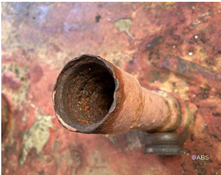
Sounding pipe closing cap thread damaged
