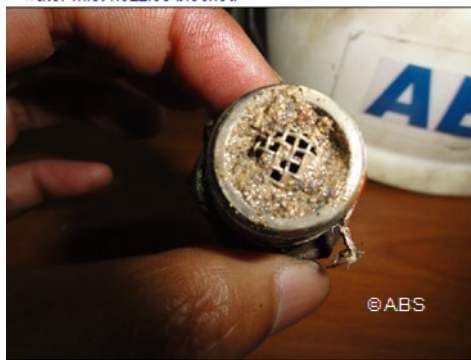
Water mist flexi fog system unable to build pressure due to nozzle clogged
