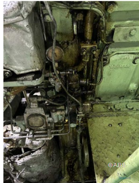
Signs of fuel leak from diesel generator engine
