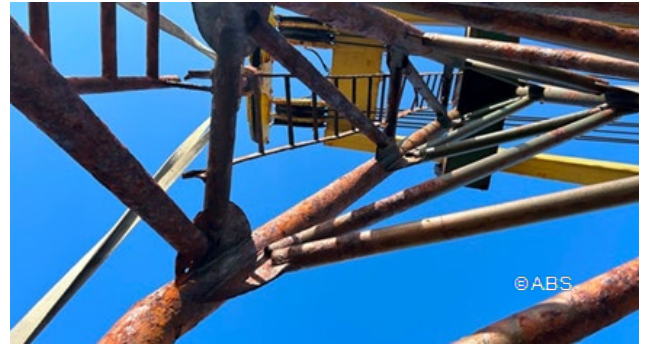
Damaged crane-rest post
