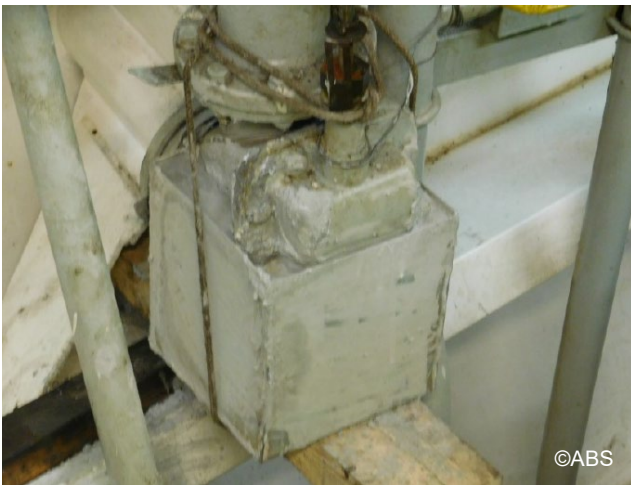
Temporary cement box repair to grey water valve
