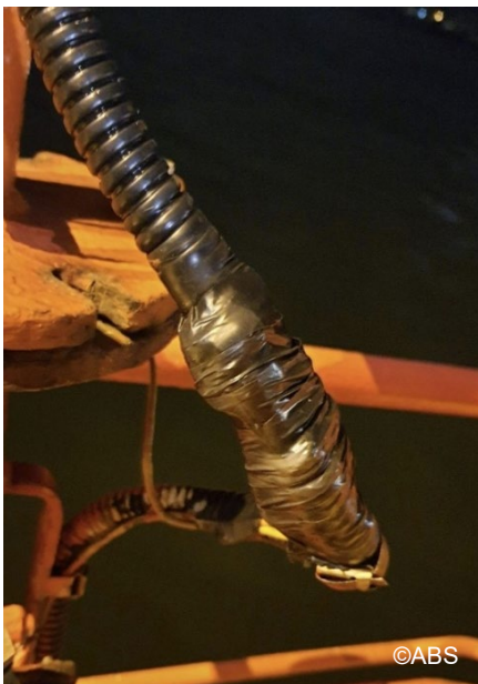
Pilot embarkation light found with electrical cables faulty
