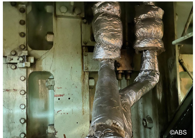
Fuel piping found without insulation – after
