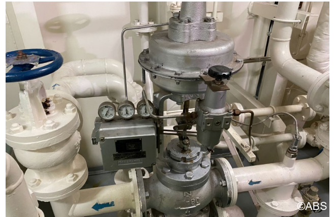
Jacket water controller cleaned after main engine propulsion control irregularity
