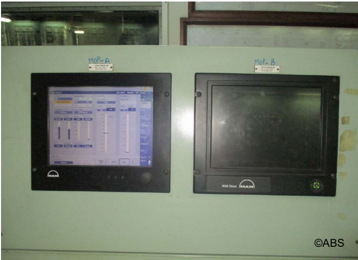
Main engine defective component for CPU replaced
