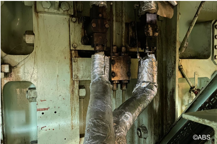
Fuel piping found without insulation - before
