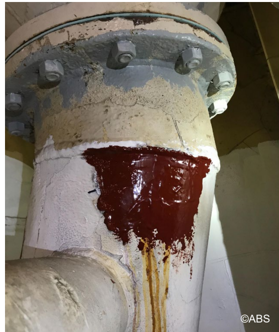
Ballast piping found with soft patch
