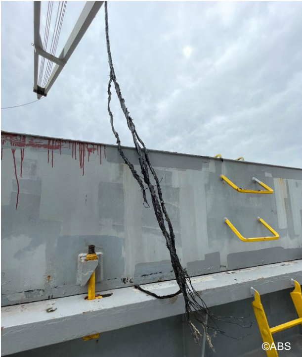
Cargo crane wire parted - before
